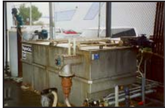
CAF Installation at a Tortilla Plant.
