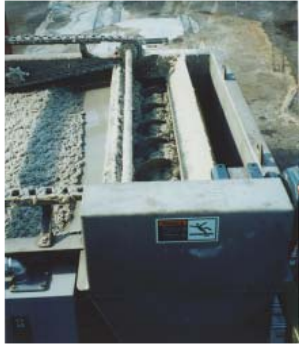
Scrapers move a thick sludge blanket to the auger area.
