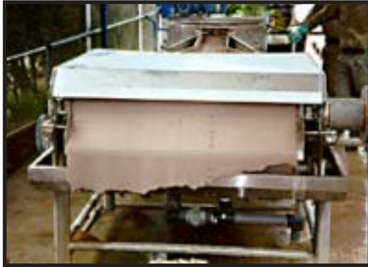
1.0 Meter Belt Press System in operation.
