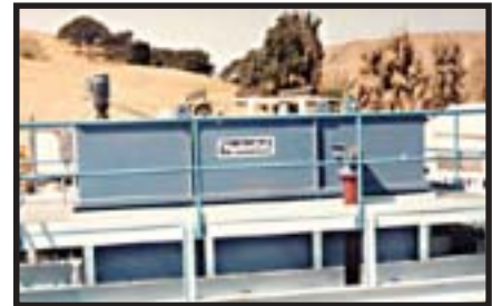
CAF-25 Installed above bio-system.
