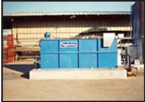
CAF unit installed at an egg ranch/plant.
