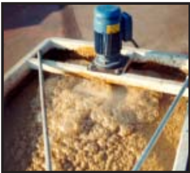
A thick layer of solids floating on the surface prior to discharge.
