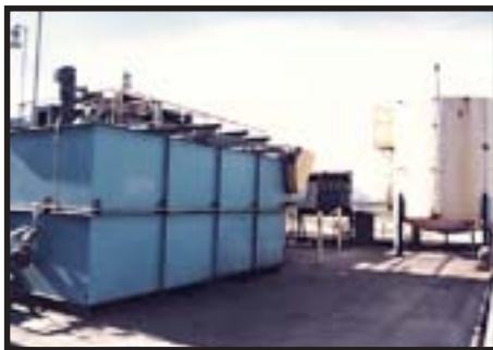
CAF unit and clarified effluent holding tank.
