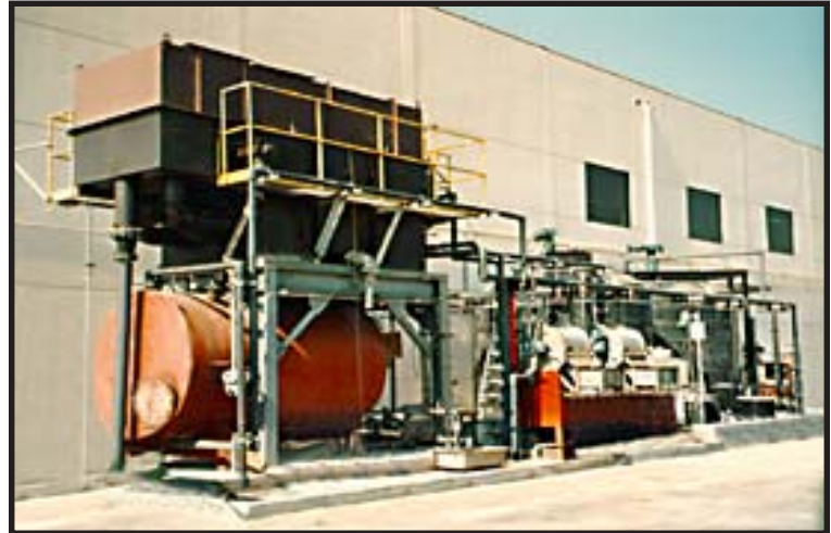
CAF-50 Flotation System installed above grade. Equalization Tanks also shown.
