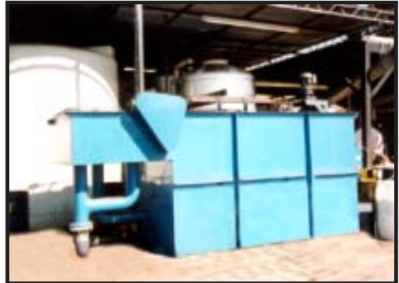
CAF-25 Installed in Industrial Laundry.
