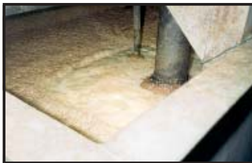
Sludge layer created by the aeration bubbles.
