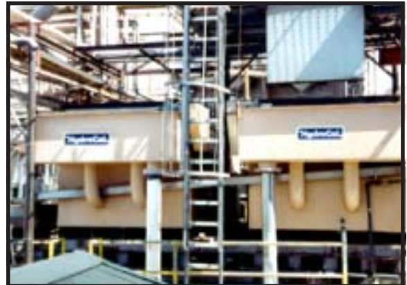
Twin CAF systems installed in an olive plant.
