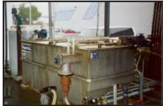
CAF Installation at a Tortilla Plant.
